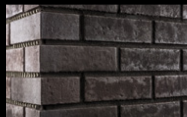
The finished joint pattern. Full masonry stretches are grouted at one go.
