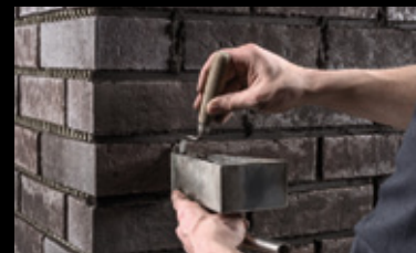
The vertical joints can be finished more easily with a smaller pointing trowel.
